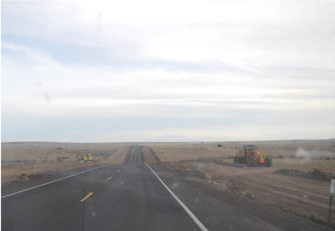
Example of ODOT constructing passing lanes on US 97 in south Sherman County (June 2015)
