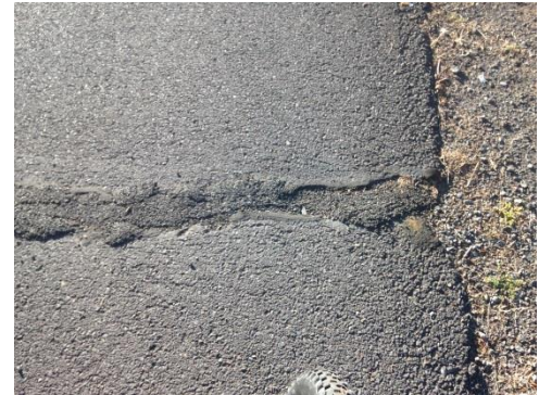
Example of crack in trail pavement
