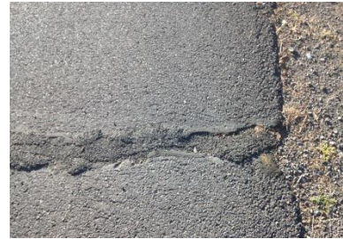
Patched Crack on OC&E Trail
