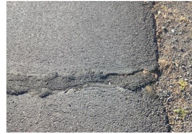
Patched Crack on OC&E Trail
