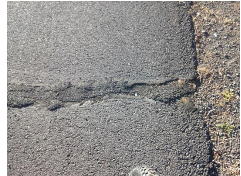
Crack in trail pavement
