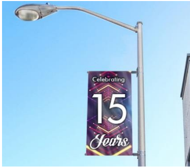
Street Lighting (with Pole Banners)
