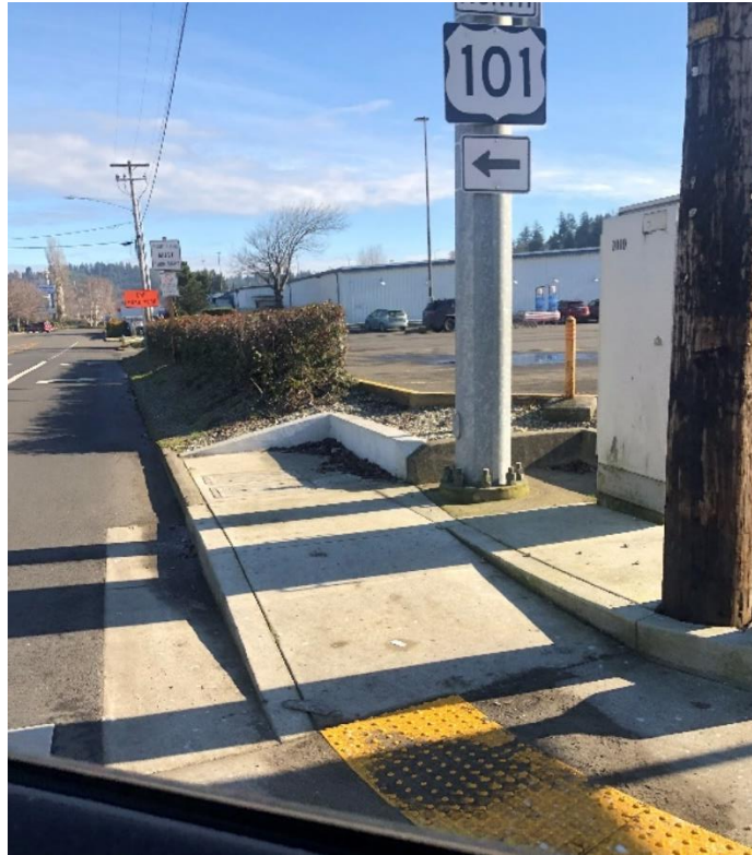
Figure 38. Lack of sidewalk connectivity on Johnson Ave, Coos Bay
